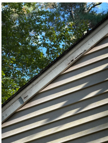
2.7 Item 1 (Picture) WDI damage
