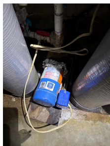
2.7 Item 16 (Picture) Leaking well pump
