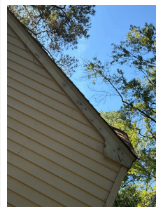
2.7 Item 6 (Picture) WDI activity and damage
