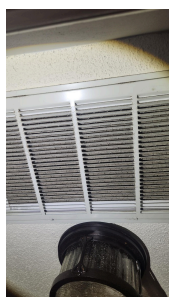
8.3 Item 1 (Picture) hallway ceiling return filter
