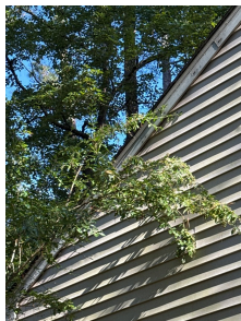
2.7 Item 2 (Picture) Overhanging vegetation
