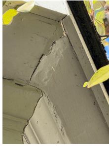
2.5 Item 2 (Picture) Rear left
