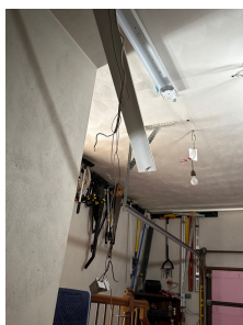
2.7 Item 20 (Picture) Damaged fixture, exposed wiring
