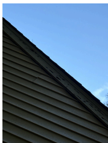
2.7 Item 5 (Picture) WDI activity and damage
