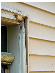
2.7 Item 8 (Picture) Moisture damage at rear
