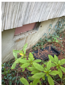
5.0 Item 2 (Picture) Rear left
