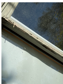
2.7 Item 11 (Picture) Moisture damage at right window
