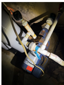
2.7 Item 17 (Picture) Corroding pump, signs of previous leaking
