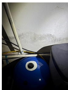
2.7 Item 19 (Picture) Dark staining at interior
