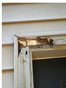
2.7 Item 7 (Picture) Moisture damage at rear
