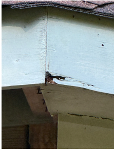
2.5 Item 1 (Picture) Rear left
