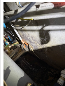
2.7 Item 18 (Picture) Dark staining at interior
