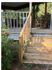
2.3 Item 2 (Picture) Rear left
