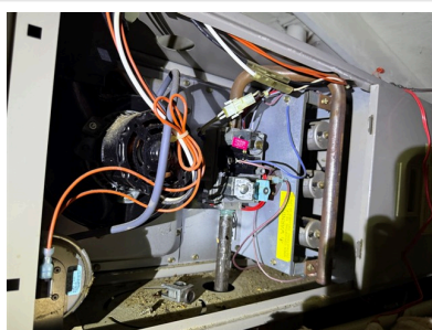
8.0 Item 1 (Picture) Furnace burner area
