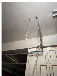
2.7 Item 13 (Picture) Removed light fixture, exposed wiring
