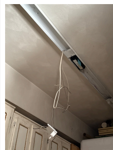
2.7 Item 12 (Picture) Damaged light fixture, exposed wiring
