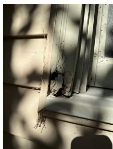
2.7 Item 10 (Picture) Moisture damage at right window
