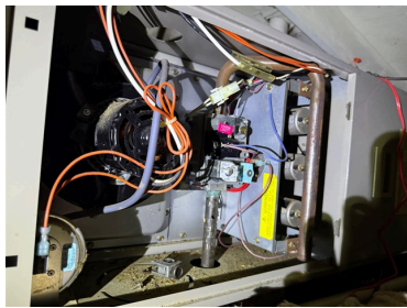
8.0 Item 1 (Picture) Furnace burner area
