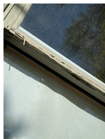
2.7 Item 11 (Picture) Moisture damage at right window
