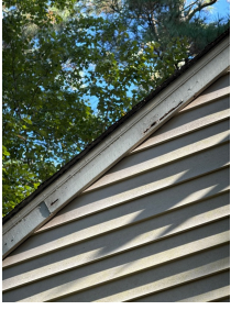
2.7 Item 1 (Picture) WDI damage
