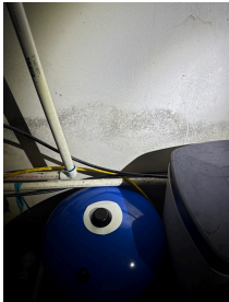
2.7 Item 19 (Picture) Dark staining at interior
