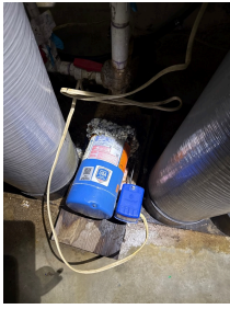
2.7 Item 16 (Picture) Leaking well pump
