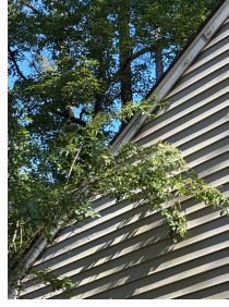
2.7 Item 2 (Picture) Overhanging vegetation
