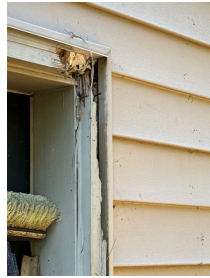
2.7 Item 8 (Picture) Moisture damage at rear
