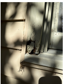
2.7 Item 10 (Picture) Moisture damage at right window
