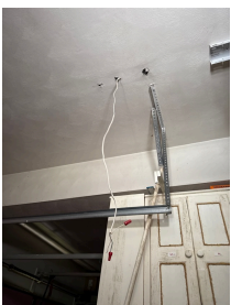
2.7 Item 13 (Picture) Removed light fixture, exposed wiring
