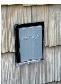
2.0 Item 1 (Picture) Rear right exterior loose siding, no J channel
