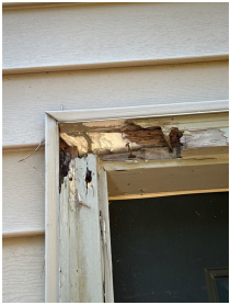
2.7 Item 7 (Picture) Moisture damage at rear
