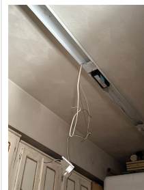
2.7 Item 12 (Picture) Damaged light fixture, exposed wiring
